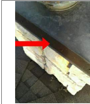
There are a few loose Nails around the chimney cap. They should be pound it in.
