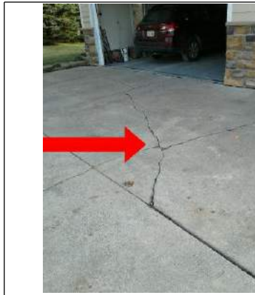
Several cracks in the cement in front of the garage.
