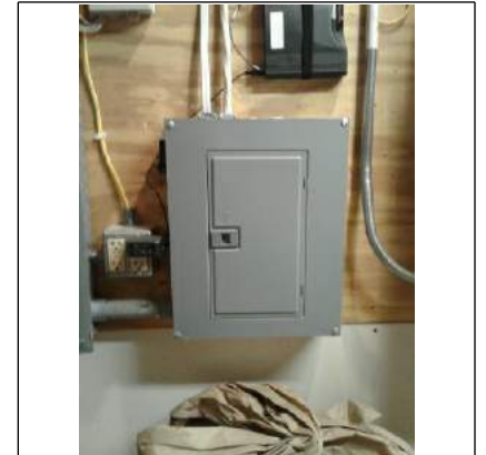
This box was put in for a generator. The generator has never been installed.
