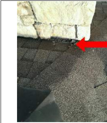
A small piece of brick maybe missing on the corner of the chimney.
